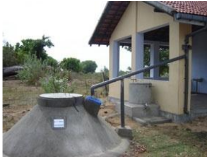
20 m 3 - partial underground tank at Maha Oya school (2)
