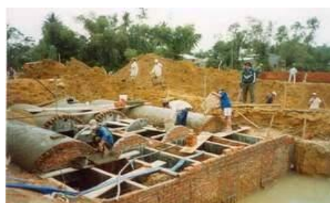
Figure 7 - Biogas digester installation in Son La
